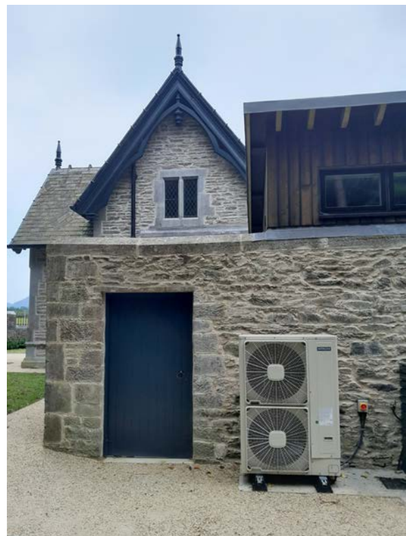
Figure 63: Air source heat pump
