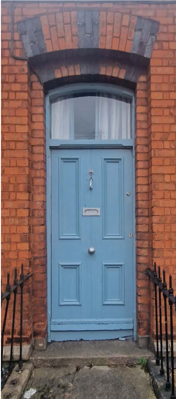
Figure 47: Aluminium draught strips can be seen to all sides of this door. Internally there is an insulated curtain
