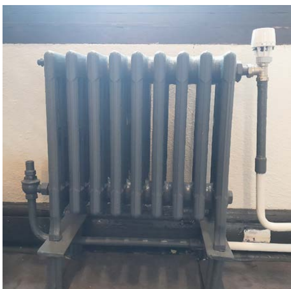
Figure 23: Cast-iron radiator with a thermostatic control
