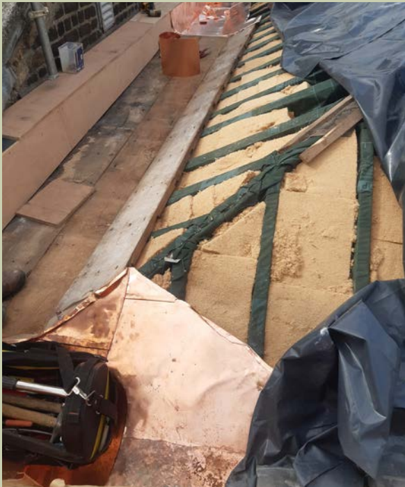
Figure 33: Wood-fibre insulating sarking board being applied between the rafters at roof level. (Image courtesy of OPW)
