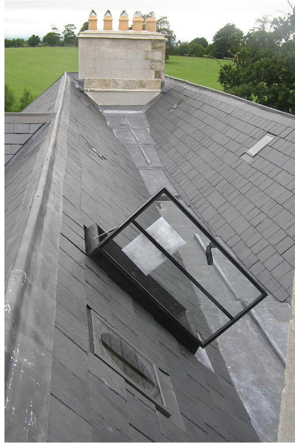
Figure 36: This modern double-glazed skylight allows access to a concealed valley gutter for maintenance inspections and cannot be seen from ground level (Image from Advice Series: Roofs , 2010)
