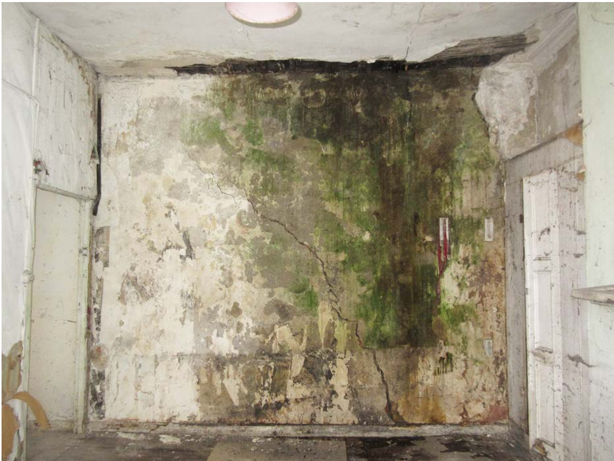
Figure 18: Extreme case of moisture ingress due to poor maintenance
