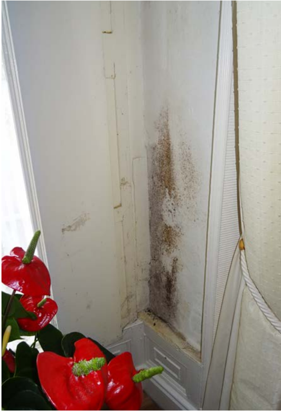
Figure 17: Mould growing behind shutters
