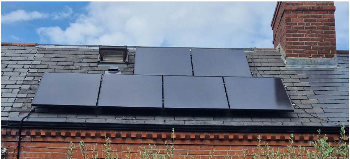
Figure 66: PV on the front roof pitch of a traditional building
