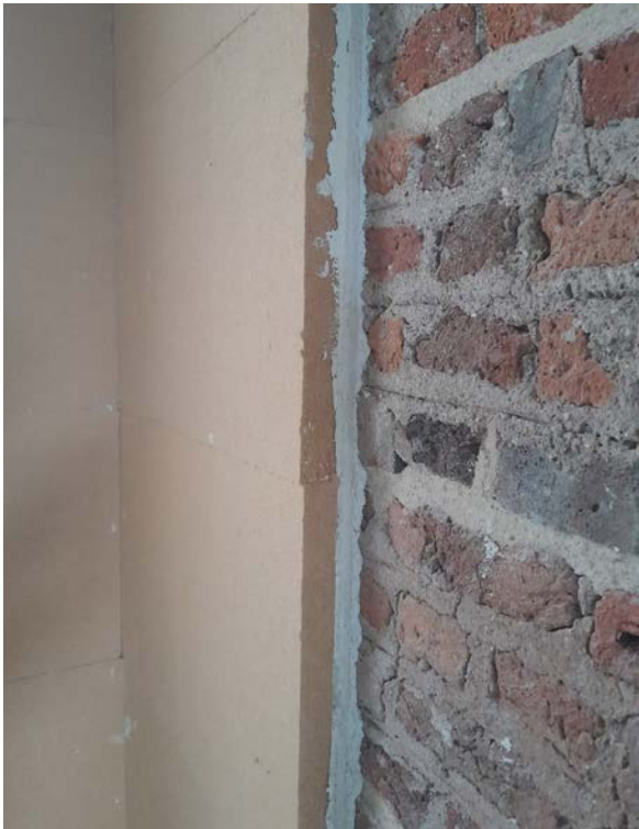
Figure 55: A layer of lime mortar is applied to the wall to provide a level surface to which to fit the woodfibre board
