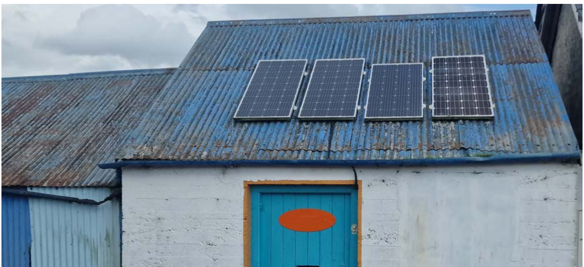
Figure 67: PV on the roof of an outbuilding
