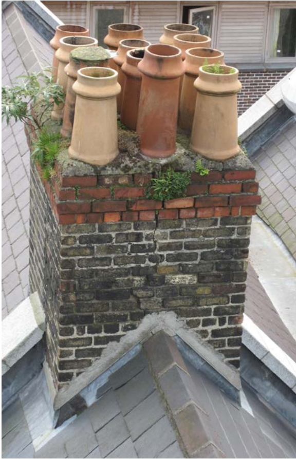
Figure 35: Traditional chimney stack requiring repair and maintenance
