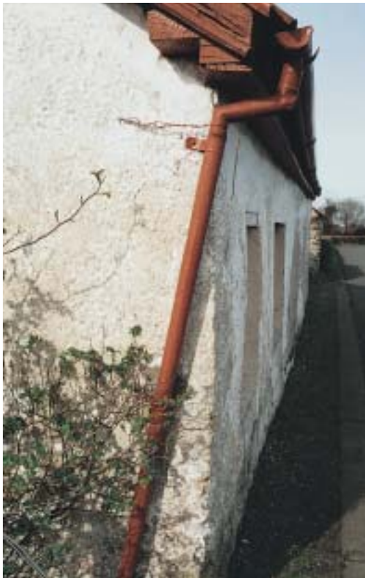
Badly set gutter – the tilt should be away from the building.
